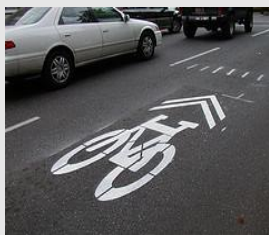
Shared lane markings: Placed on 'normal' roads where bicycles share traffic lanes with motorised vehicles.
